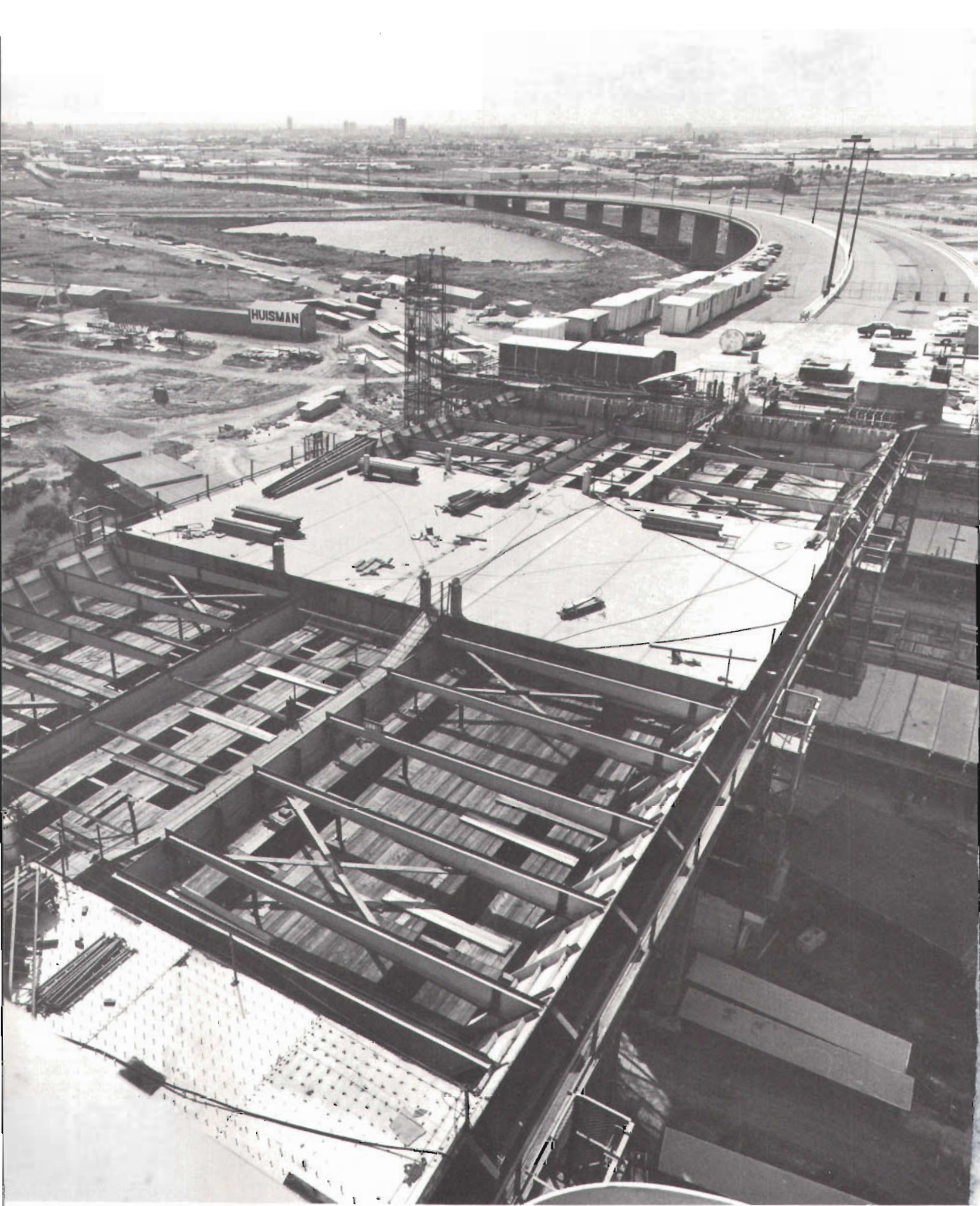
Replacement of top deck panels and strengthening of erected steelwork on the east side. The substantially complete East Approach Viaduct and the Toll Plaza are shown in the background.
